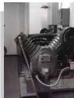
Air Compressor – Full Visible
