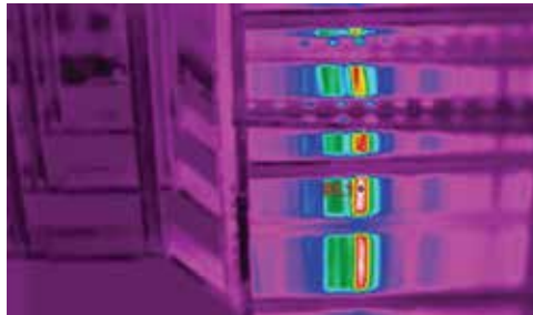
Overheat on power bar caused by unbalanced load. 橋架動力電纜由於負載不匹配導致過熱
